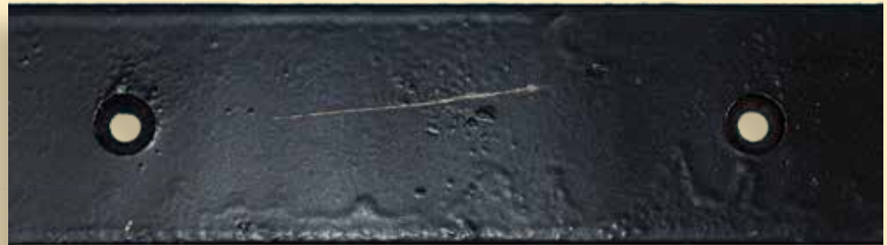
Close up of Deliberate Scratch shows little rust, no rust migration, and no detachment of the surface coating
